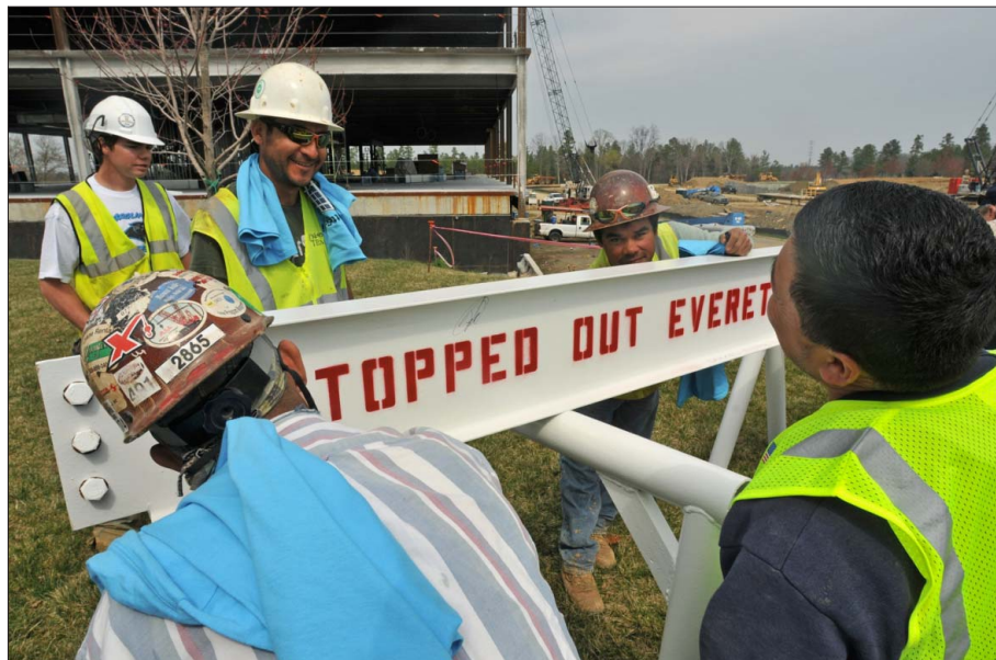
Workers sign the last steel beam to top out the Everett building, the latest "spec" office structure going up in Bissell Cos.' Ballantyne Corporate Park, despite the recession. The building, named for civic activist Mac Everett, is on North Community House Road.
