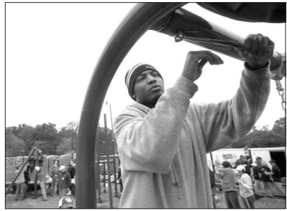
TODD SUMLIN - tsumlin@charlotteobserver.com James Jackson tightens bolts on a new swing set at Paw Creek Elementary School. Hundreds of volunteers came out for the 10th annual event, which builds a new playground in one day.
